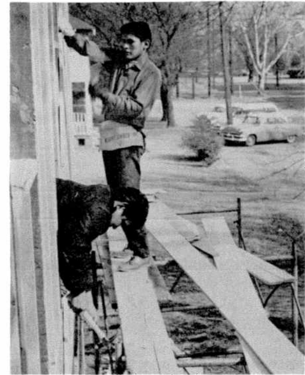
Clark Josley and Billy Blackwater are shown here working on a new apartment building soon to be occupied by employees.
