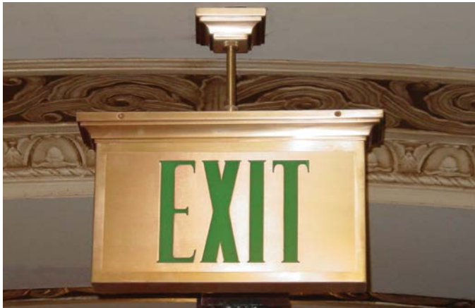
Figure 13. Careful selection, design, and location of exit signs can help preserve the historic character of significant historic spaces while still meeting code requirements. Photo: Marilyn Kaplan
