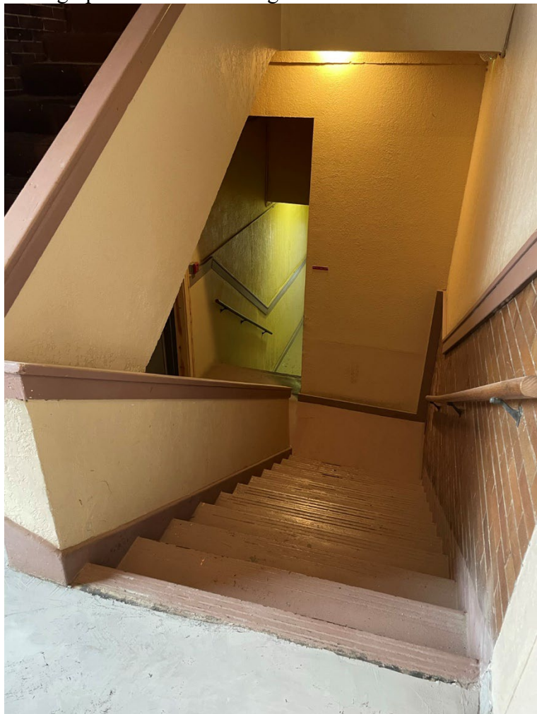
Photograph 10: Interior image of interior stairwell from the first floor to the basement level.
