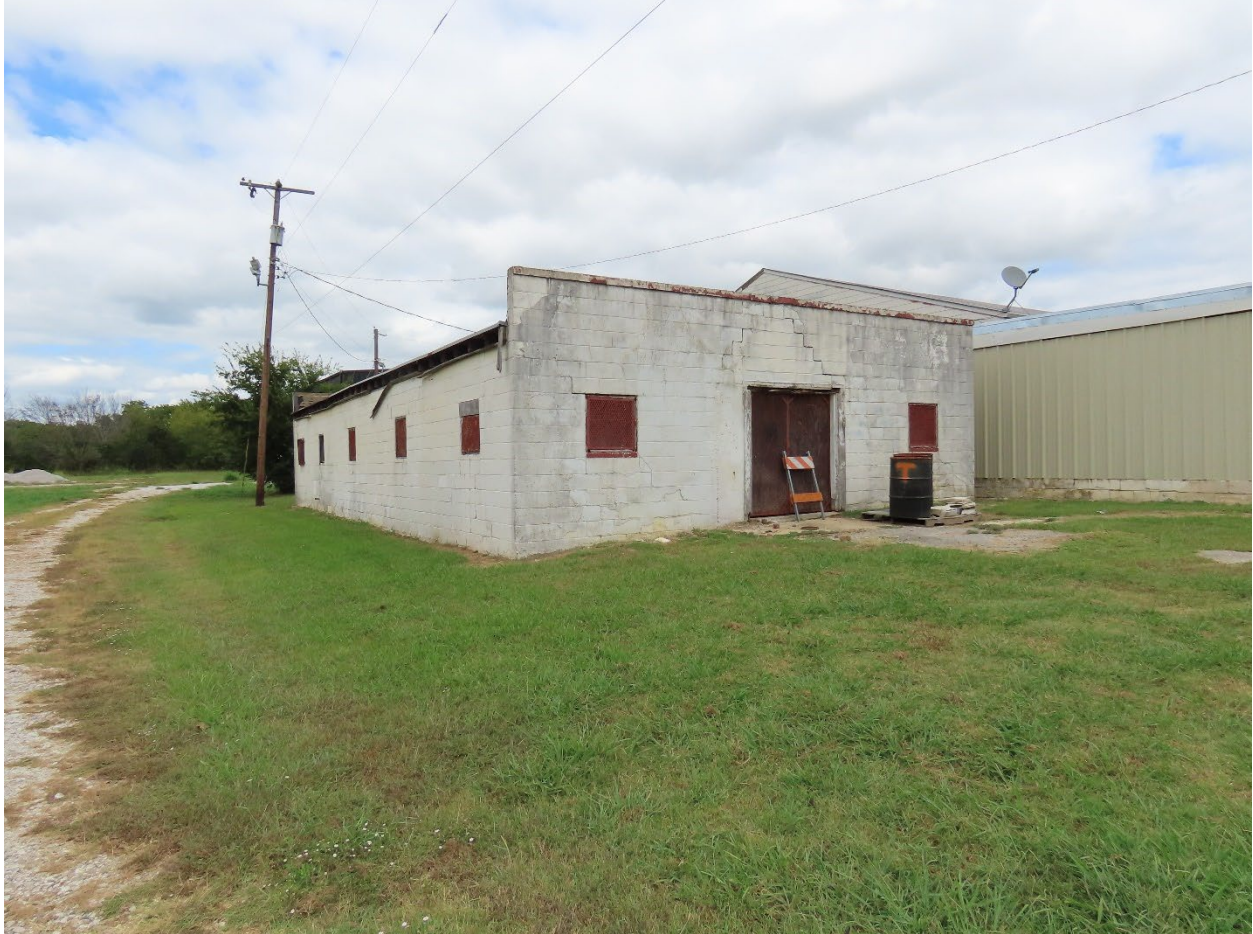
Photograph 30. Oblique of Moton School Shop south façade and west elevation, facing northeast
