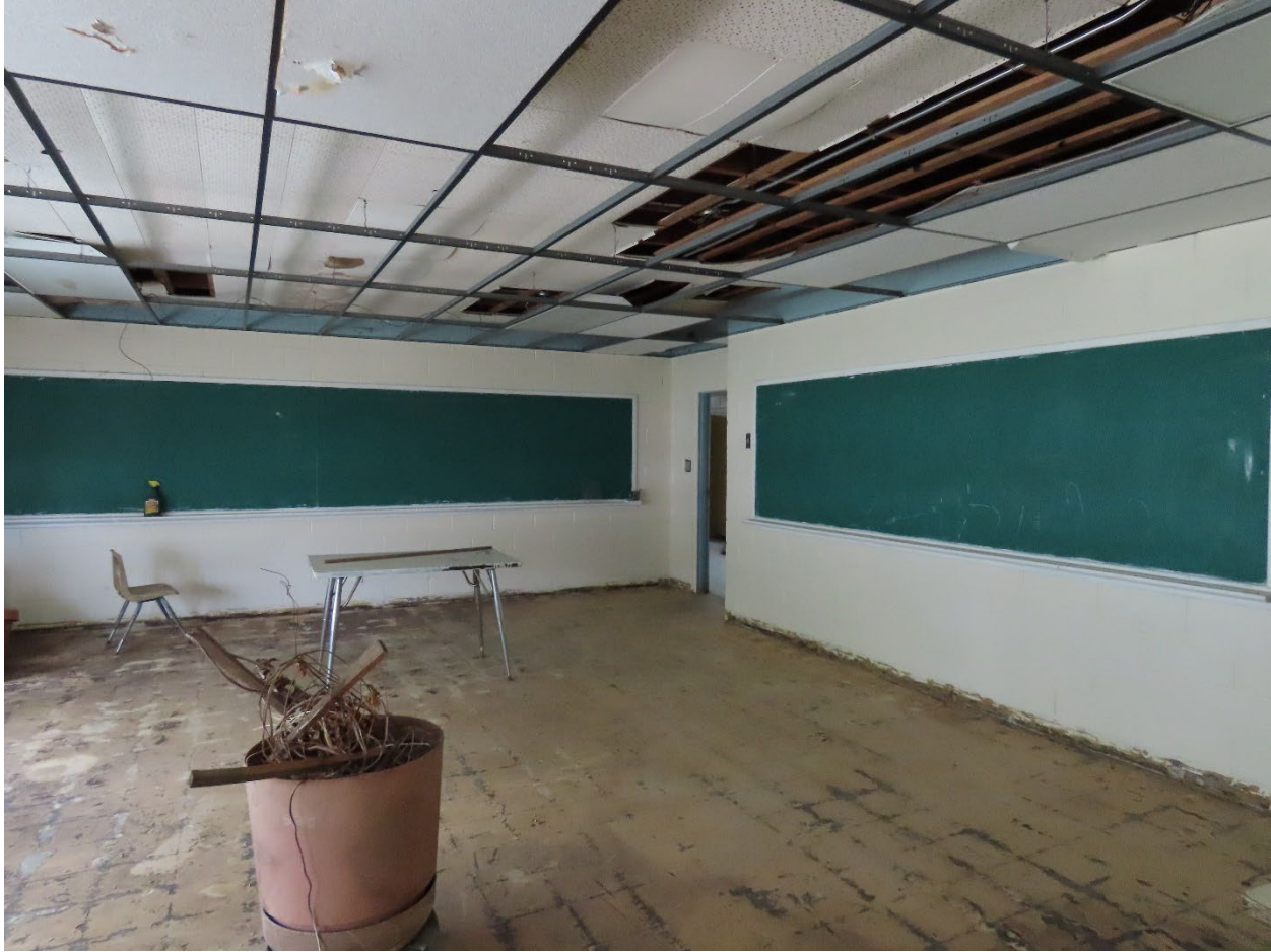
Photograph 17. Interior of Moton High School classroom with two chalkboards, and some flooring and some drop ceiling removed, facing southwest
