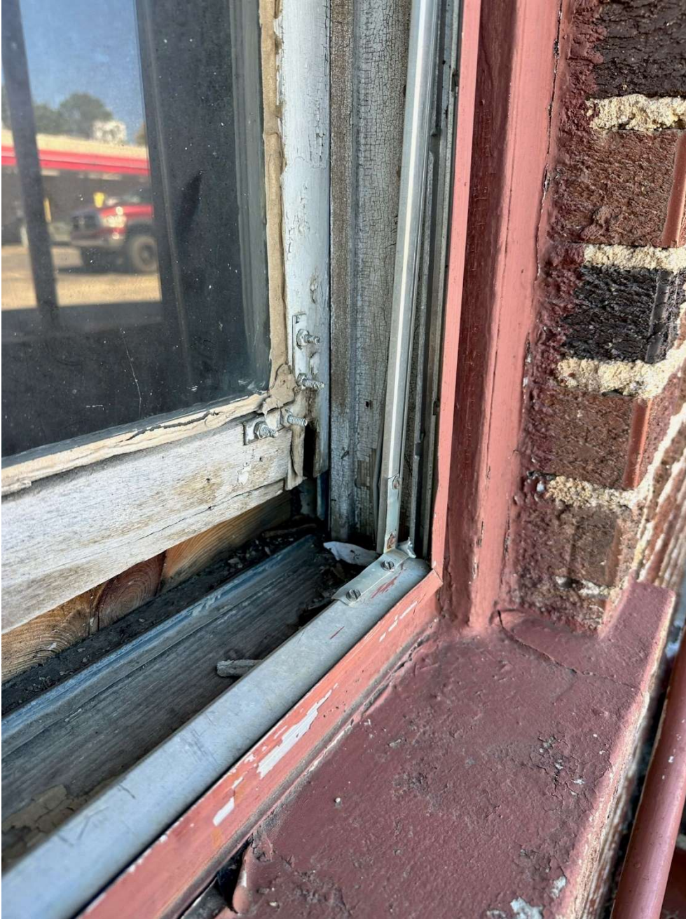
Original window at the Van-Sanford Apartments. All the original windows are non-operational. Photo taken looking southwest.
