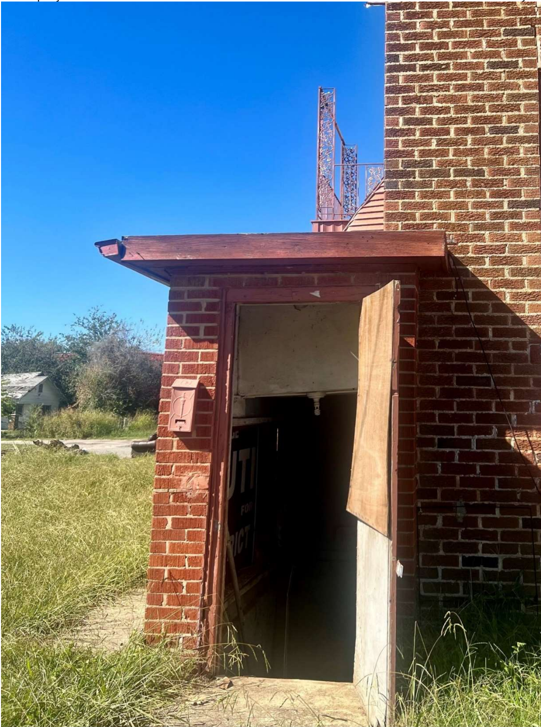
East façade of the Van-Sanford Apartments, showing the front view of the corner side entrance that leads to the basement. Photo taken looking west.
