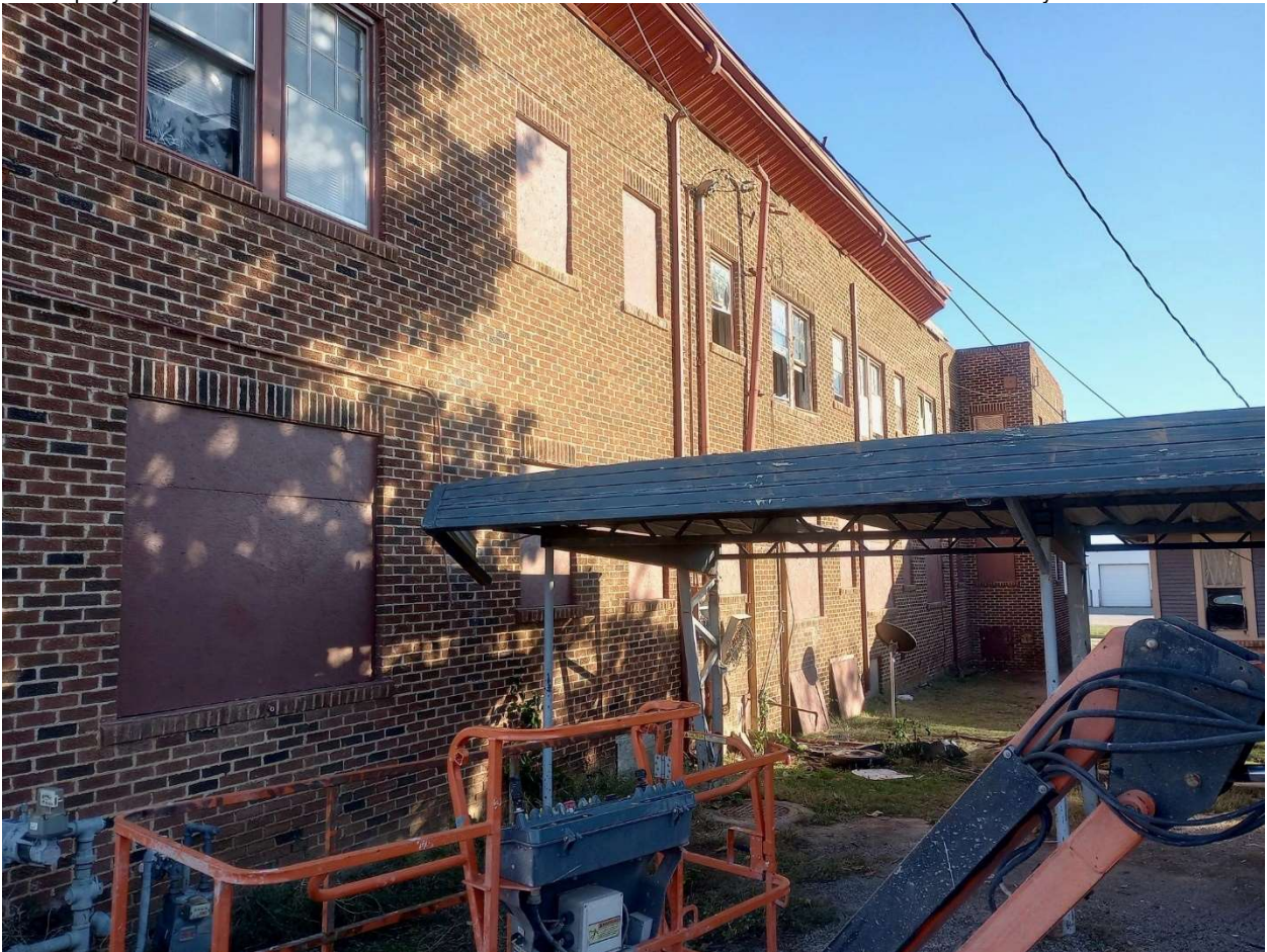
West façade of the Van-Sanford Apartments, showing the back side of the building. Photo taken looking southeast.
