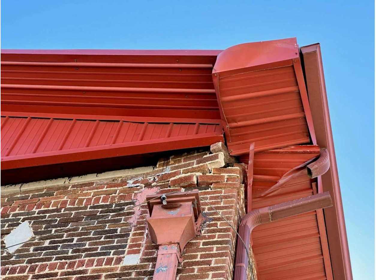
Damage caused to the parapet wall due to the installation of the metal roof on the Van-Sanford Apartments sometime in the late 1980s. Photo taken looking up and south.
