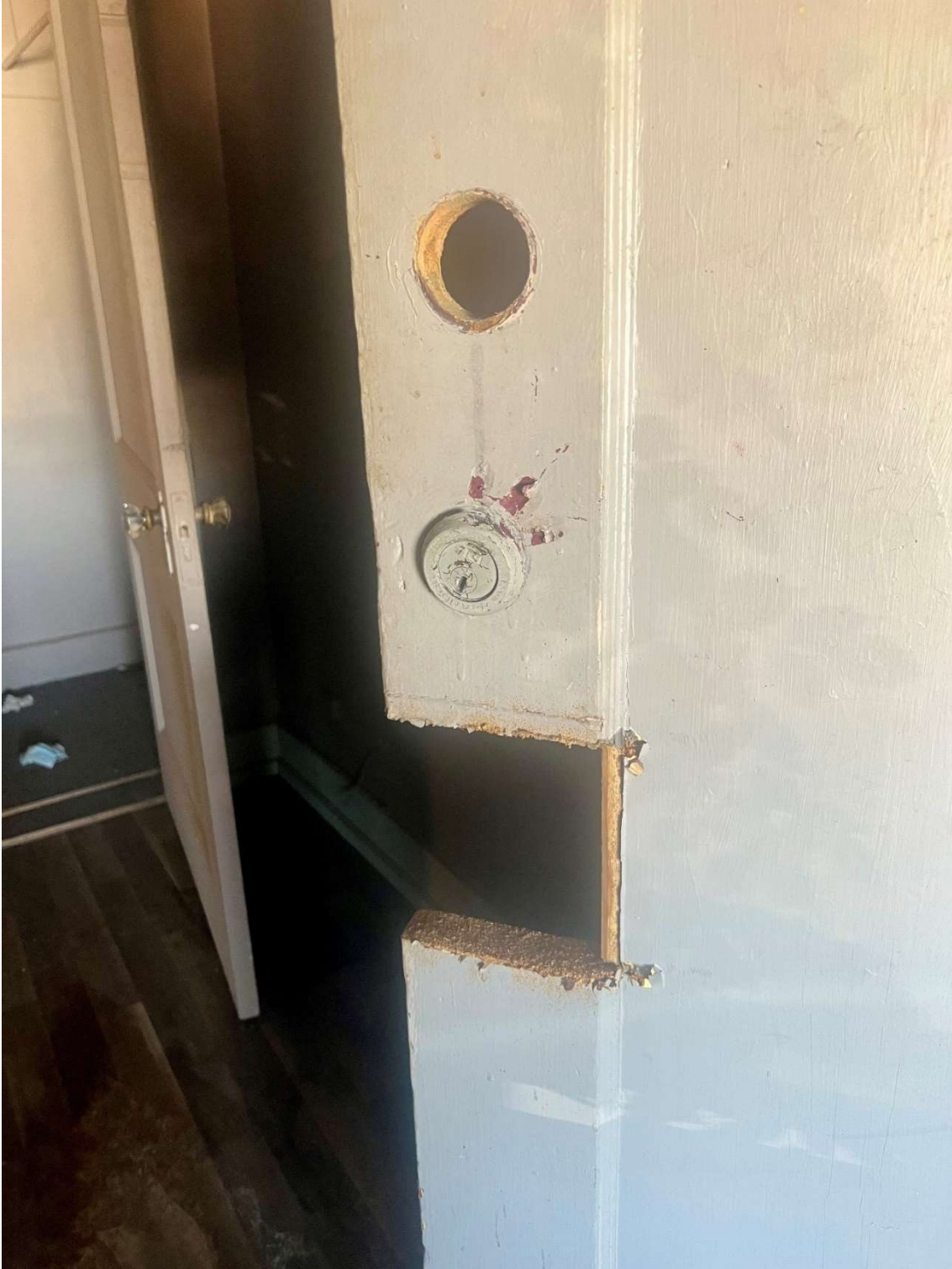
Damage to an interior door inside the Van-Sanford Apartments caused by vandalism when the building was left vacant after the tornado of May 2022.
